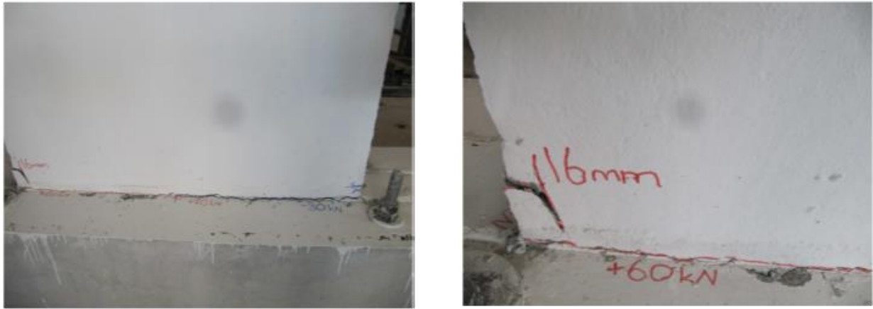
Figure 7. Cracking patterns of SW at 16 mm lateral displacement
