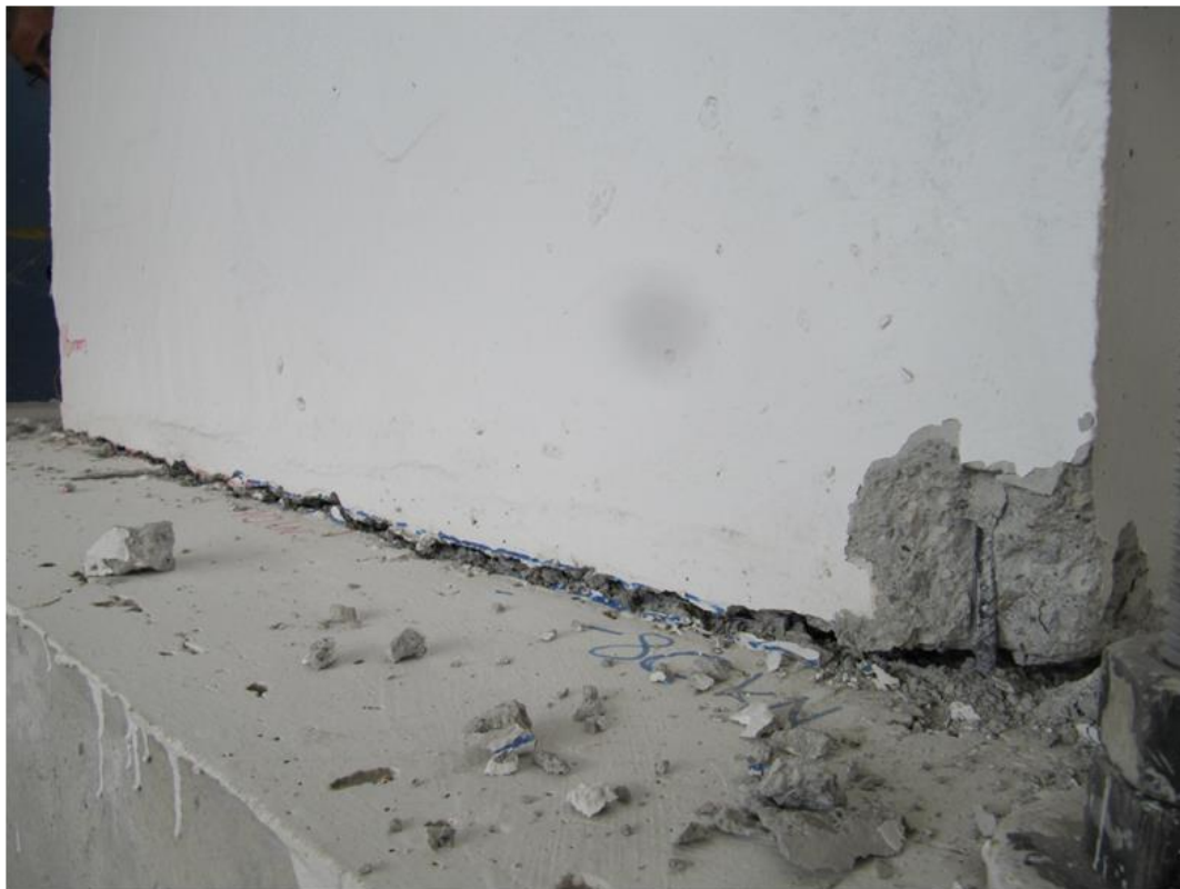
Figure 9. Overall condition of SW test specimen at end of test
